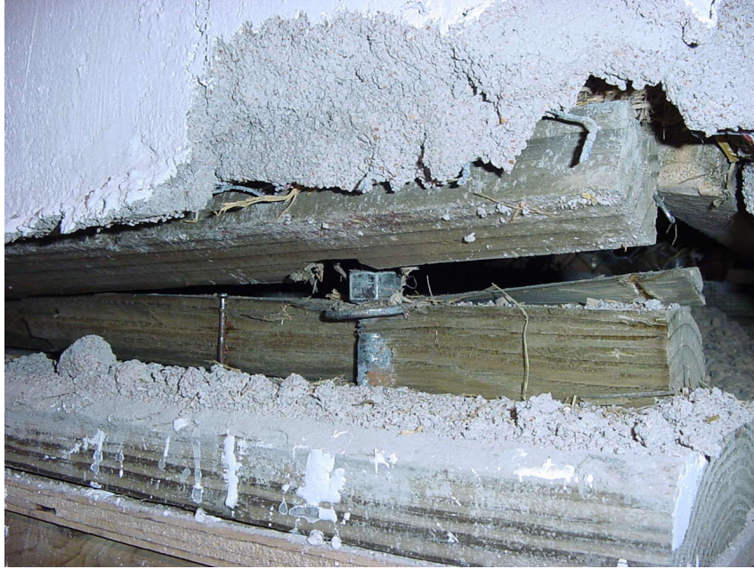
Figure 6.6 – Wall D cross-grain bending failure of sill plate (Photographed at 5% drift, well after failure had occurred)
