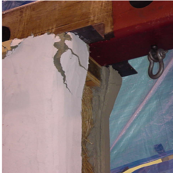
Figure 6.2 – Evidence of header beam slippage in Wall A
